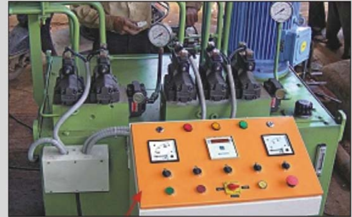
Fully Automatic Control Panel
